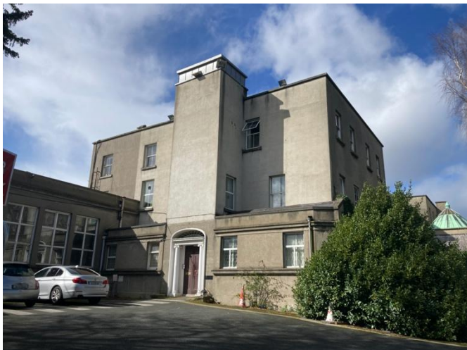
Plate 7.3.23: Present day connection of the truncated Finlay Wing with Milltown Park House
