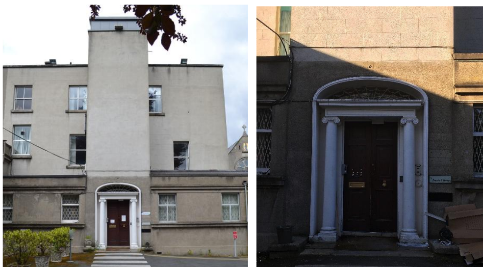
Plates 7.3.15 & 7.3.16: East (front) elevation of Milltown Park, with a detail of the original entrance door and fanlight within a much-altered context
