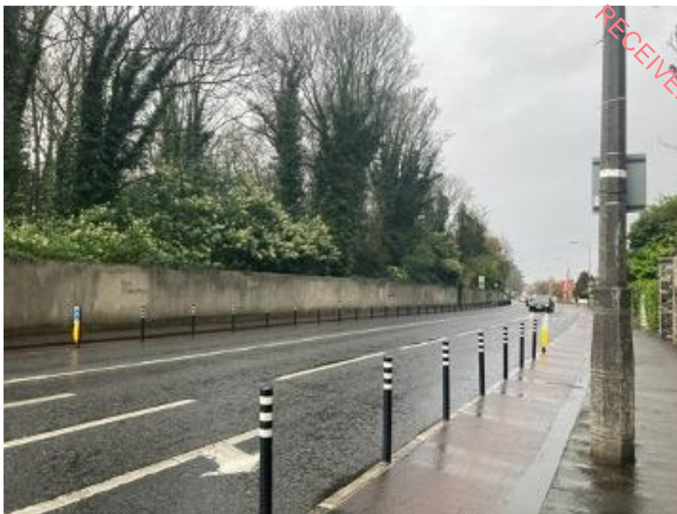
Plate 7.3.33: Section of boundary wall at junction of Milltown and Sandford Roads, due northwest which was replaced with blockwork in past realignment of the junction
