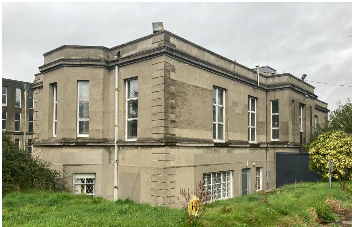
Plate 7.3.21: The front elevation of the Finlay Wing as viewed from the south
